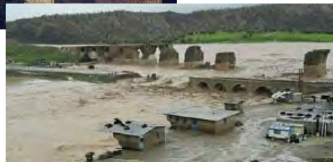
Kaskkan bridge in IRAN, affected by floods March 2019.
